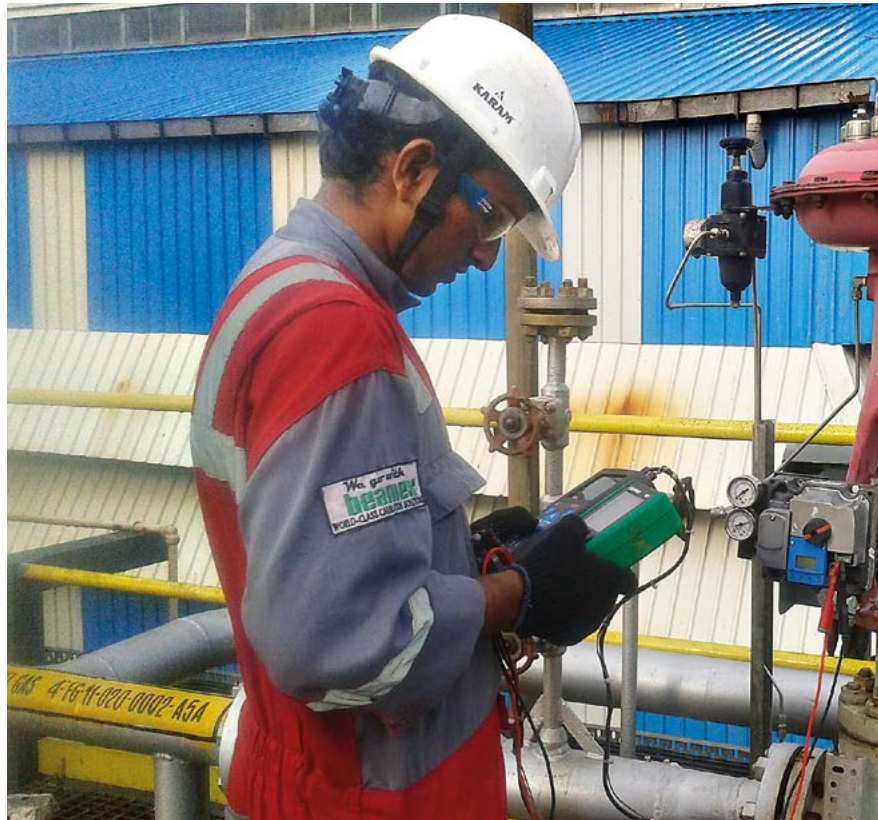
An Engineer at L-Tech Engineering does a field calibration / loop checking.
